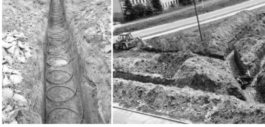
Fig. 1. Ground heat exchanger
