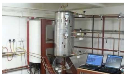
Fig. 2. Tested tube coil heat exchangers - general view of test section
