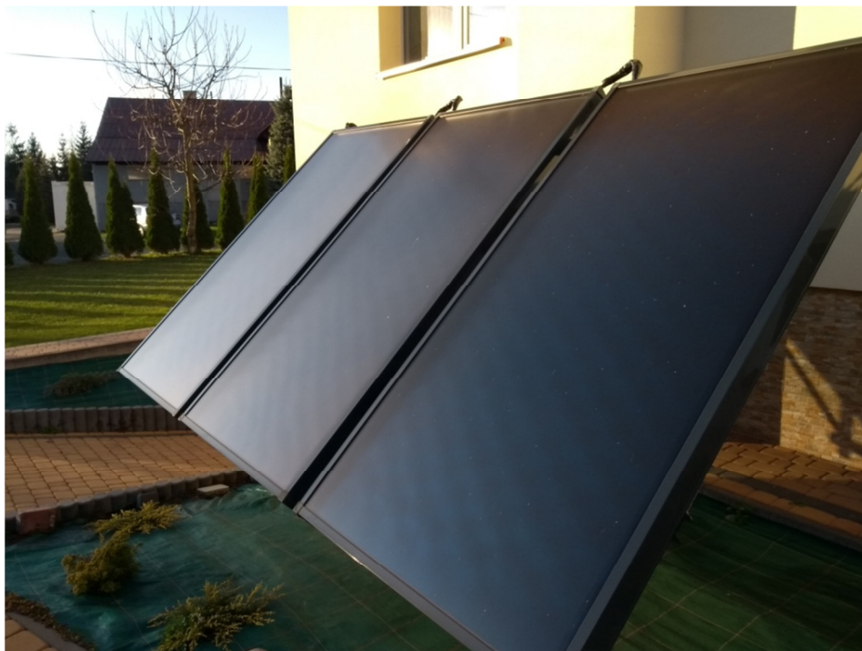
Fig. 7. Solar collectors founded on the ground, Białka. Source: own study
